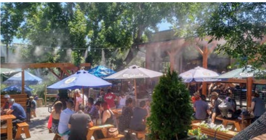
Image 12. Commercial installation of misting cooling system
