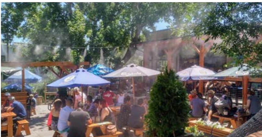
Image 2. Commercial installation of misting cooling system
