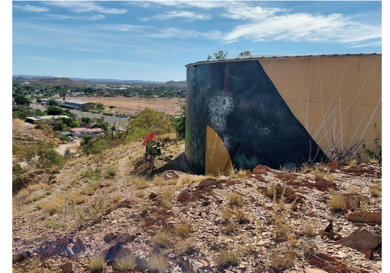
The Water Tank is unable to be viewed in its entirety unless visitors chose to go off track and walk all the way around.
